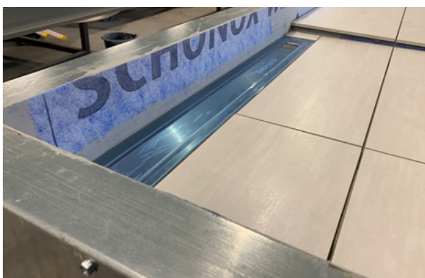
A Schönox waterproofing system installed in a bathroom pod
