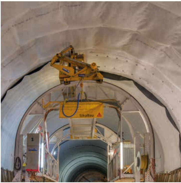
To protect the tunnel structure from water ingress, SikaBau AG, as the contractor, utilized the SikaProof®-200 in a drained waterproofing system.
