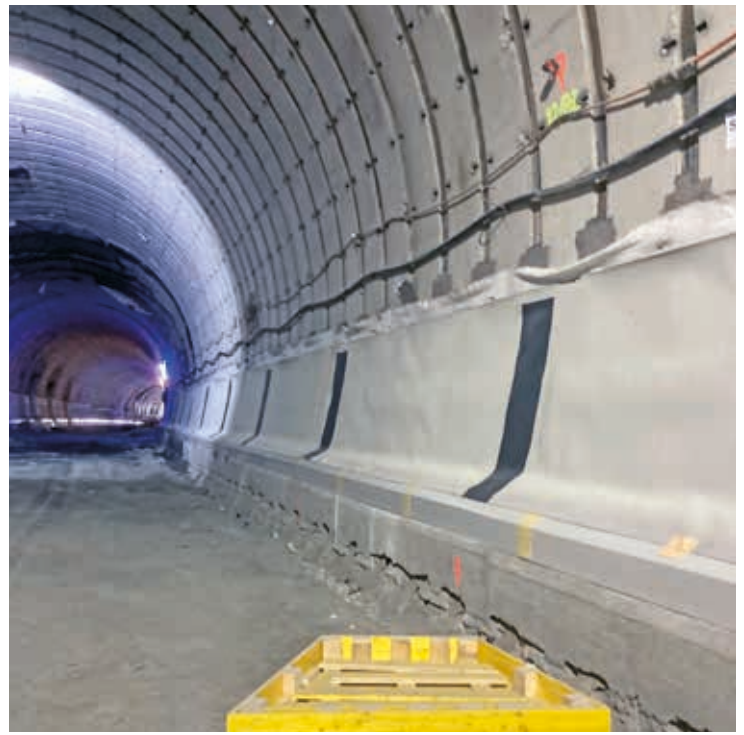
In spring-summer 2022, Sikaplan® WP Drainage Angles were installed, followed shortly after by the bottom part (kicker) of the drainage layer and SikaProof®-200.
