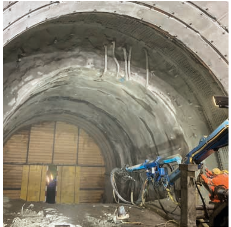
In spring 2017, excavation work resumed with elaborate reinforcement using steel beams and reinforced in-situ concrete rings. The profile in the already excavated section was widened.
