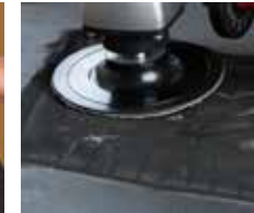
Grind the repair area edges (45-deg slope) with a tungsten sander at < 5,000 rpm
