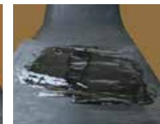
Leave and allow the correct time for the repaired area to cure
